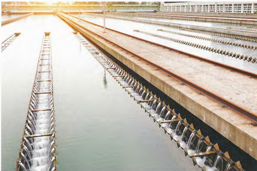
LEFT: a water treatment plant in China. As of the end of 2012, there were 3,340 sewage treatment plants in China, with a total treatment capacity of about 142 million cubic metres per day
